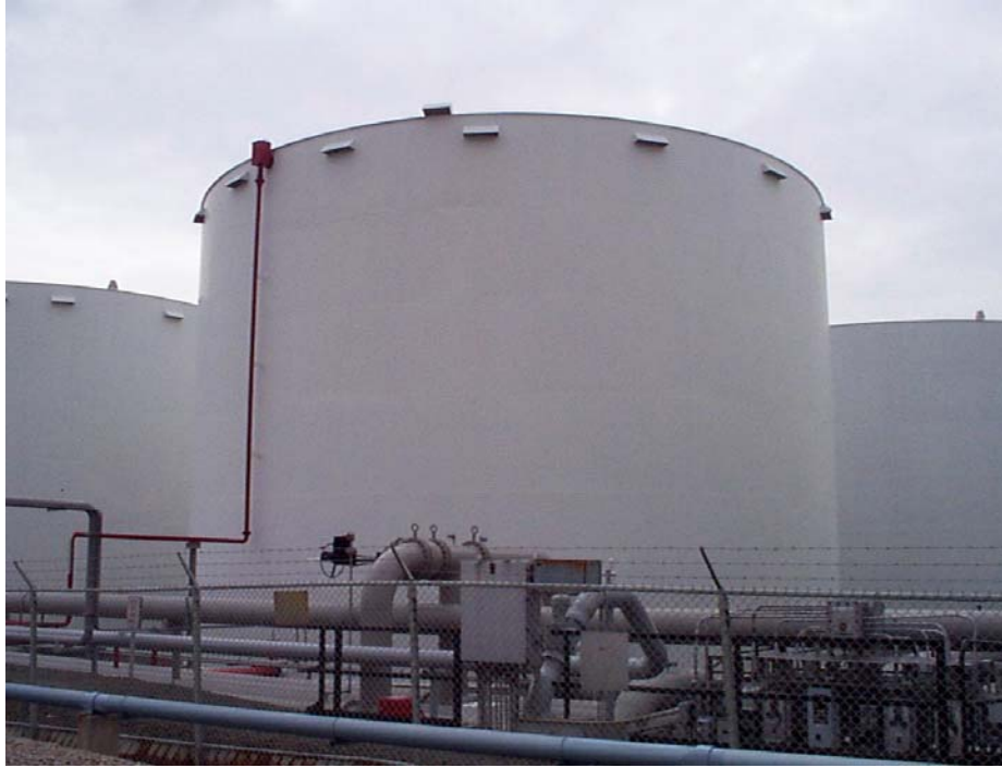
Figure 4 – 1: Cone Roof Storage Tank
